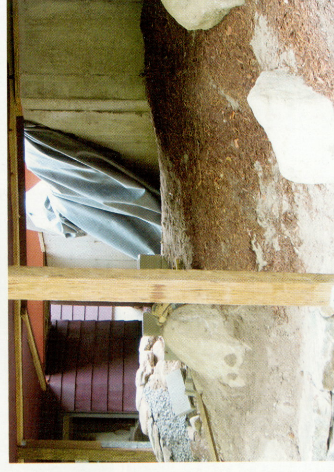
Building a pond and stream beneath a completely constructed room was the major challenge for this project. From the start, the team took their time to do everything properly.
